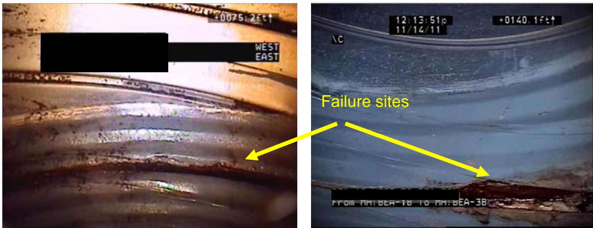
Figure A-14: Snap shots of a video from inside a pipe with severe corrosion of plain corrugated galvanized pipes.
