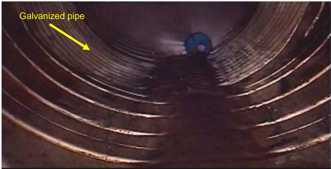
Figure A-13: Snap shot of a video from inside a pipe that shows plain corrugated galvanized pipe is joining the segments of SRAP.
