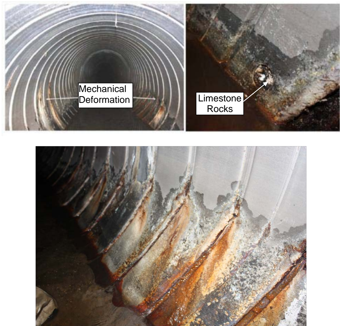
Figure 15: Photograph of in situ pipe located in Jacksonville, near Highland Glen and Beach Blvd. Mechanical damage (Top-left and bottom). Limestone rocks present beneath the bore location (Top-right).
